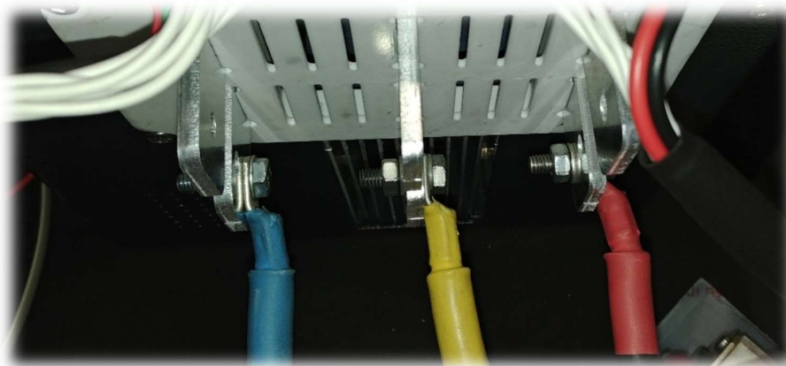
Figure 21 – Power wiring on the soft starter
